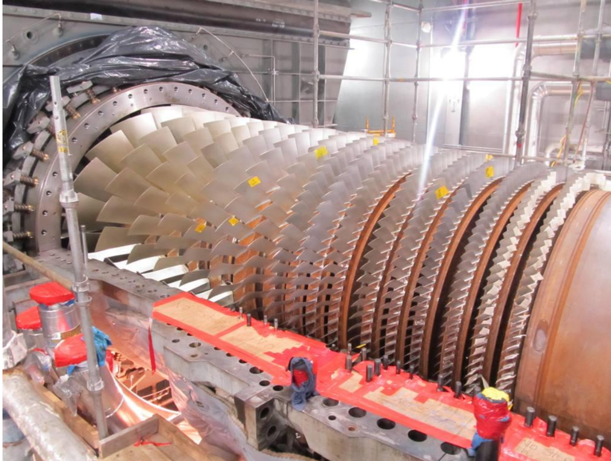
CT2 Compressor Section
